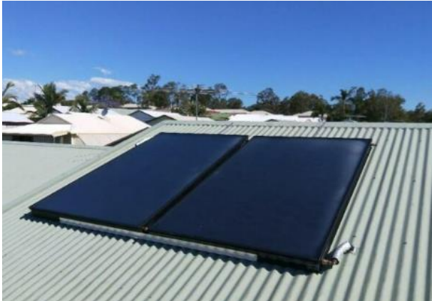
Figure 1: Solar Panel on a roof
